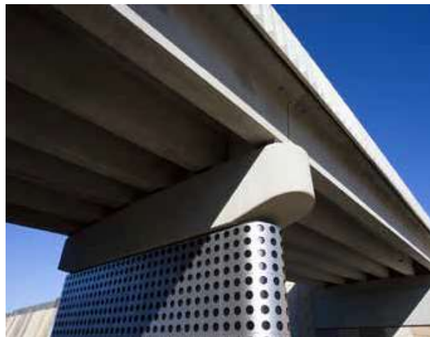
A notable early infrastructure project for New Touch Industries entailed the production of stainless steel skins for Melbourne's EastLink motorway.
